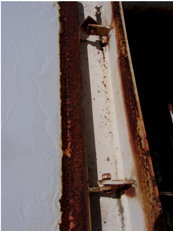
Photo #: 17 Description: Exterior Roof: Corrosion areas on the interior cover lid and adjoining curb for the Roof Access Manway.
