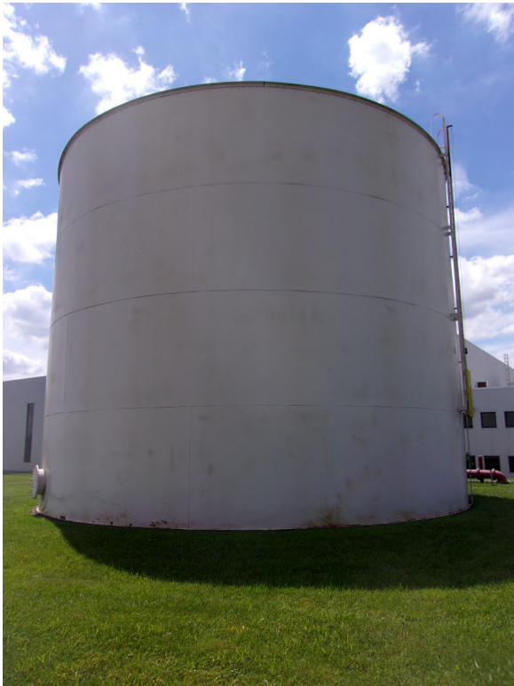
Photo #: 43 Description: Exterior Shell: General corrosion areas visible on all four (4) shell courses.
