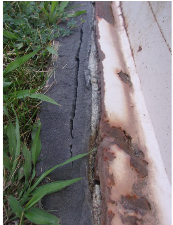
Photo #: 56 Description: Exterior: Tar sealant application cover chime/fiberboard joint has failed. Spalling concrete observed.
