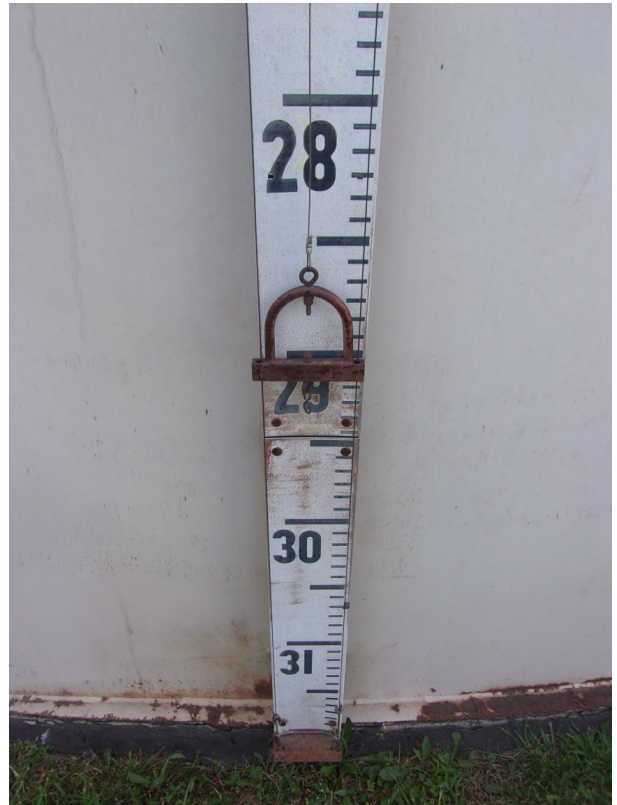
Photo #: 52 Description: Exterior: Water Level Indicator Assembly.
