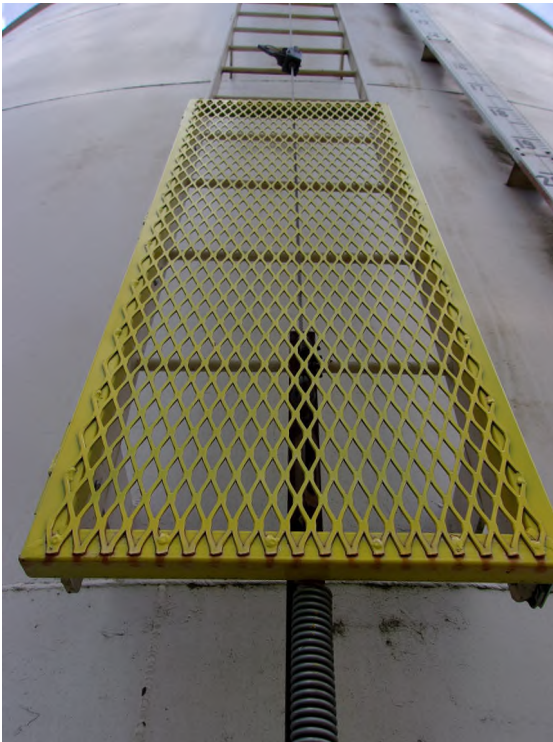
Photo #: 3 Description: Exterior Shell: View of the Exterior Access Ladder. Ladder has a framed diamond style wire, hinged, locking cover gate over the lower five (5) feet of the ladder.
