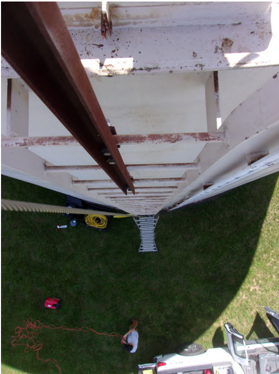
Photo #: 7 Description: Exterior Shell: Downward view of ladder rungs and shell. Upper attachment bracket for cable safety climb device is shown.
