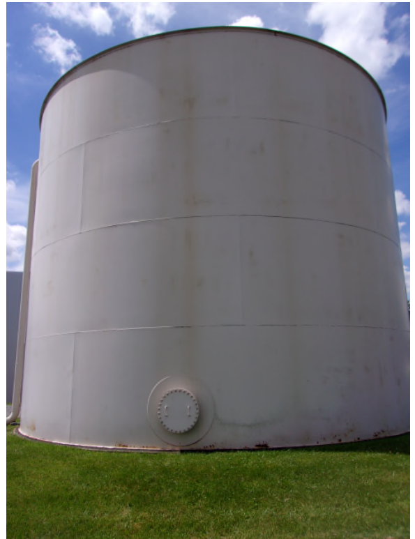
Photo #: 44 Description: Exterior Shell: General corrosion areas visible on all four (4) shell courses.
