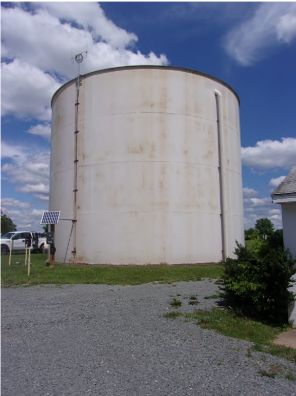
Photo #: 51 Description: Exterior Shell: General corrosion areas visible on all four (4) shell courses.
