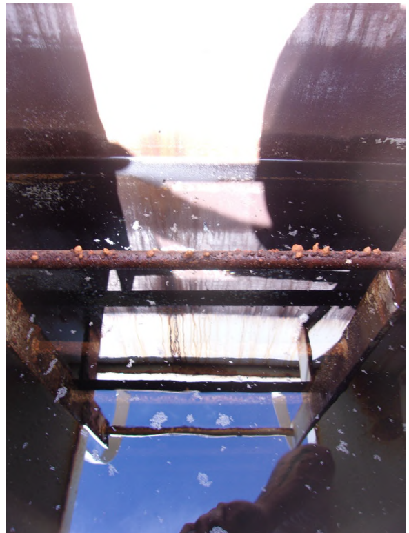
Photo #: 20 Description: Interior Wet: Close-up view of moderate to severe corrosion on the ladder rungs.
