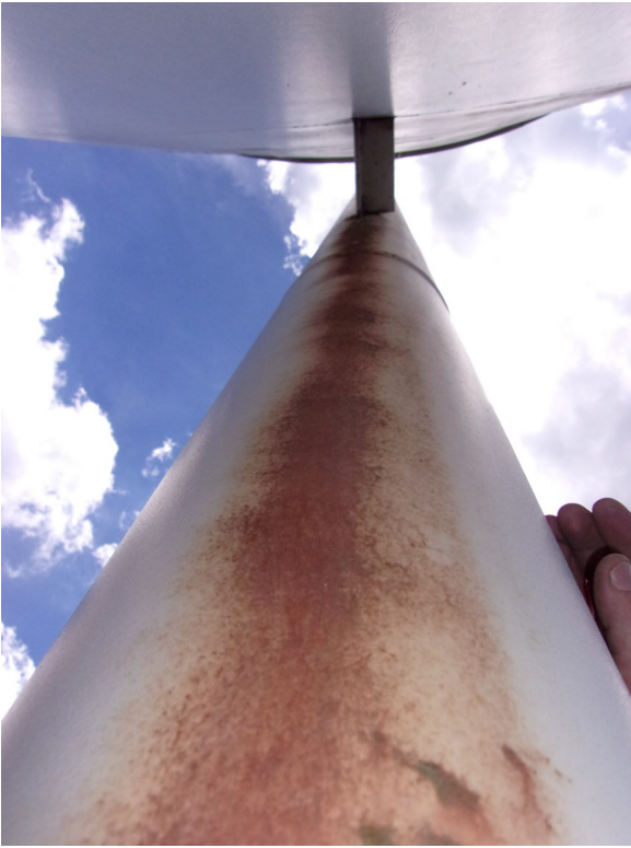
Photo #: 49 Description: Exterior: General corrosion area along the backside of the overflow pipe.
