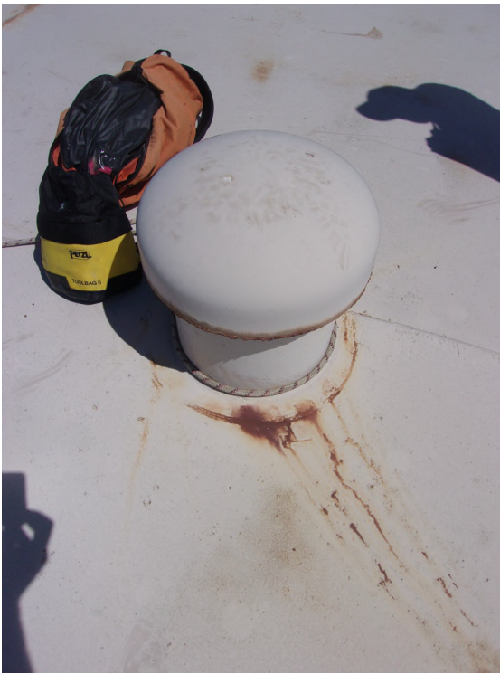
Photo #: 29 Description: Exterior Roof: Center Roof Vent. Unknown device appears to have formed a circular corrosion area on the roof plate around the neck of the roof vent.
