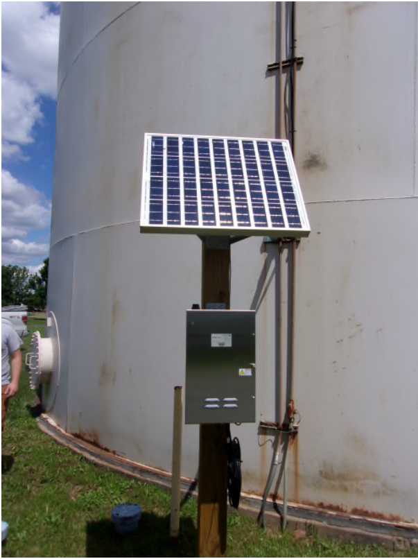
Photo #: 41 Description: Solar Power Equipment Unit.
