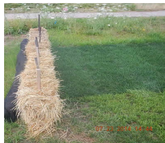
Straw Bale Barrier: Two Stakes per Bale with bale entrenched and backfilled
