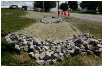
Rock Check Dams: VDOT #1 Stone or Class I Rip Rap can be used
