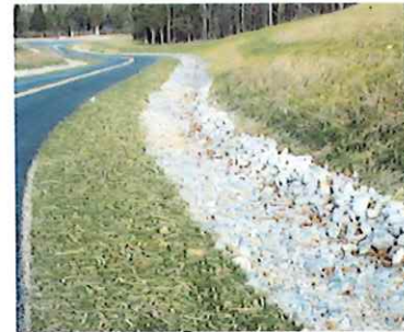
Stormwater Conveyance Channel: Channels can be grass, rip-rap, or concrete. Used to convey water away from property
