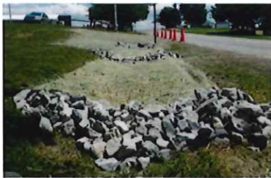
Rock Check Dams: VDOT #1 Stone or Class I Rip Rap can be used
