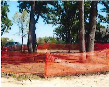
Tree Protection: Safety Fence installed around the drip line of trees to protect the root system
