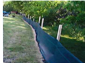
Silt Fence: Stakes should be at least 5' long and spaced no more than 6' apart
