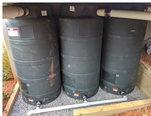
Three 300 gallon cisterns
