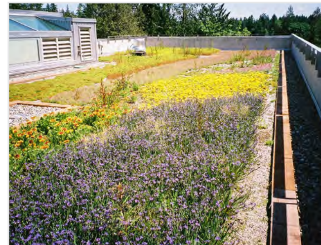
Green roofs offer biodiversity, a natural habitat and beauty while providing environmental benefits.
