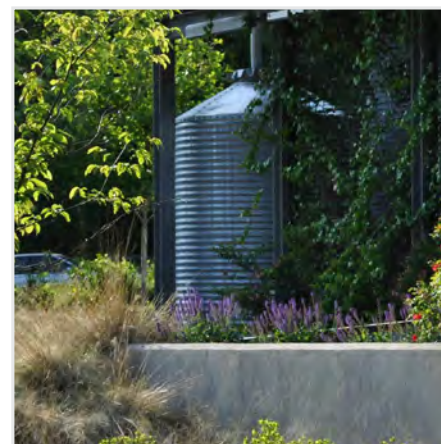
Rainwater harvesting tank, collecting water directly from the roof.
